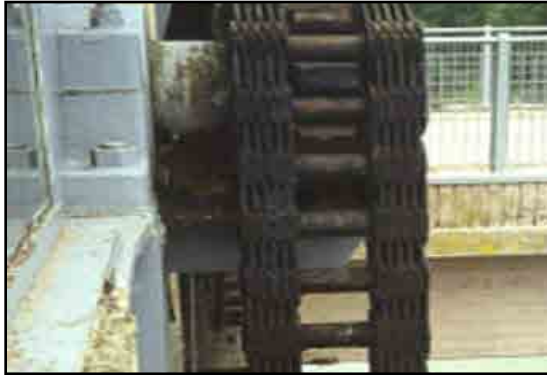
The chain was heavily contaminated.
